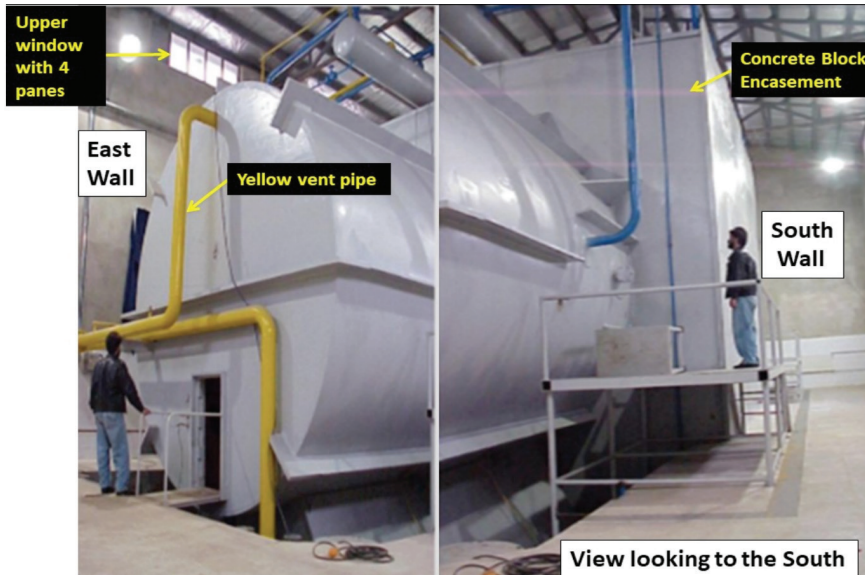
The main high explosive test chamber in Taleghan-1 Image credit: Institute for Science and International Security
